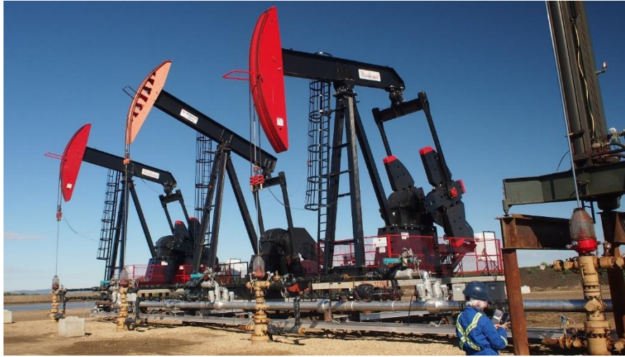
Figure 5: Well Site Guard units installed on the field.
